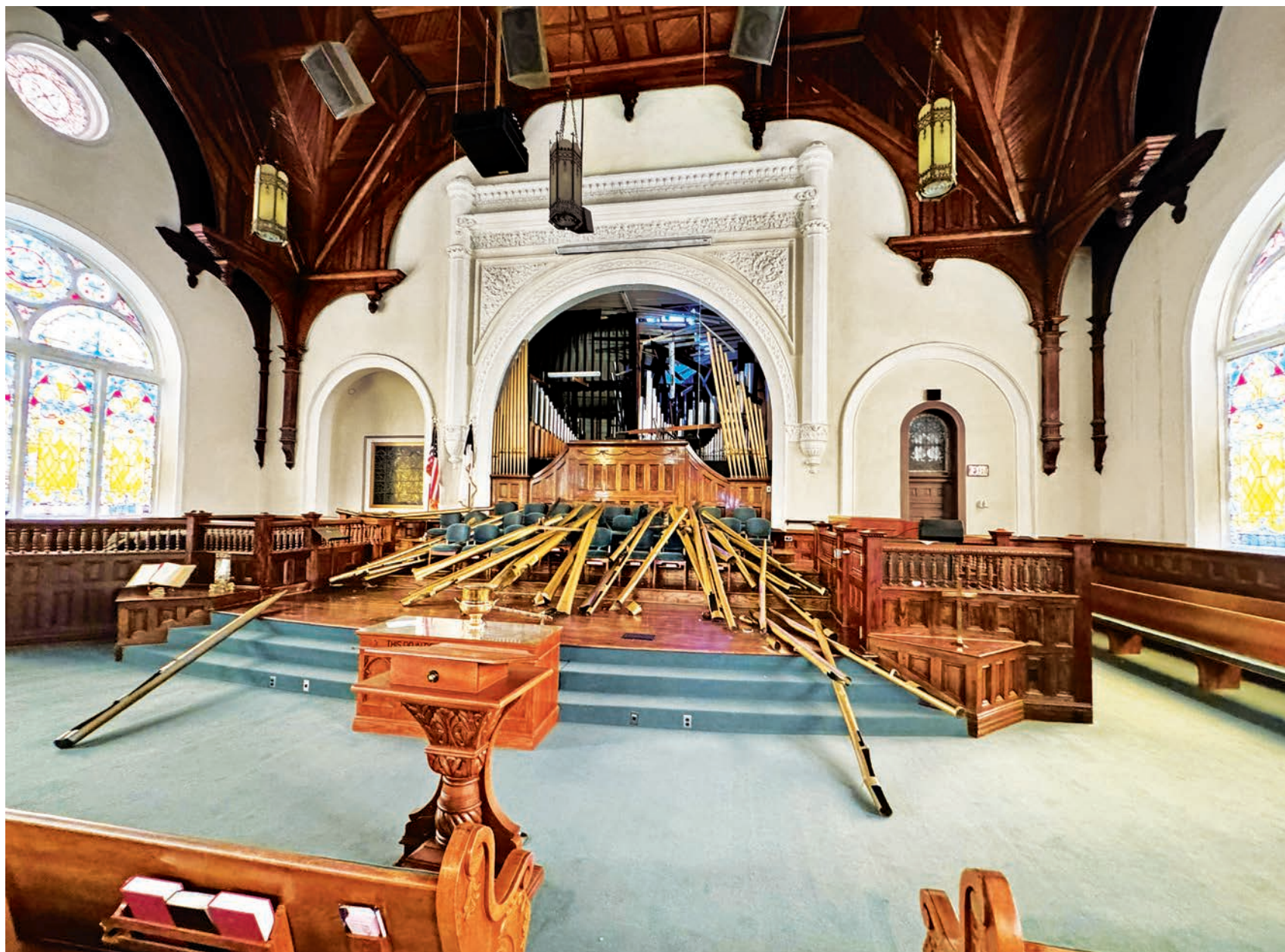
Damage to organ and façade from collapsing chimney
